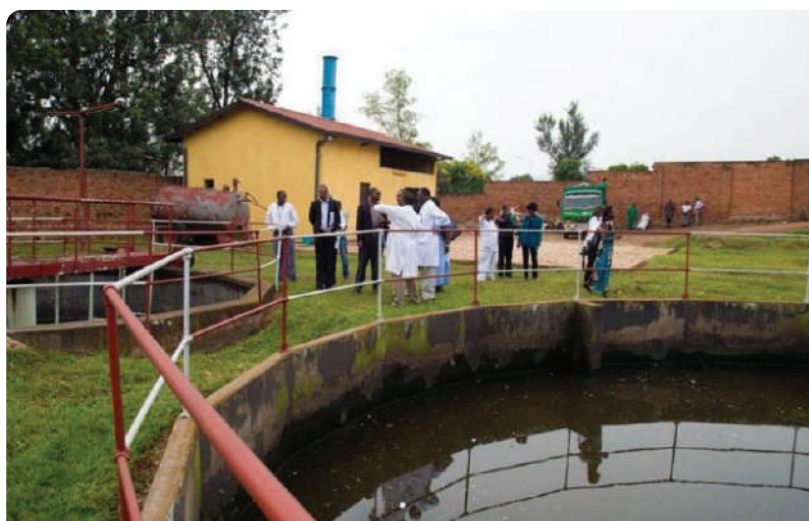
Fig 5.6: Sewage treatment plant in kigali city
